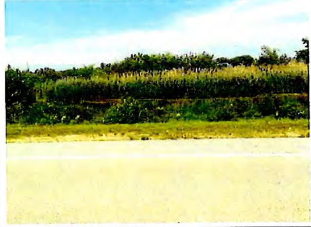
Steep shoulders with a body of water near the roadway. The water and steepness of the slope are partially hidden by tall grass.
